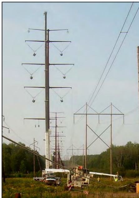
Arrowhead-Weston Transmission Line
